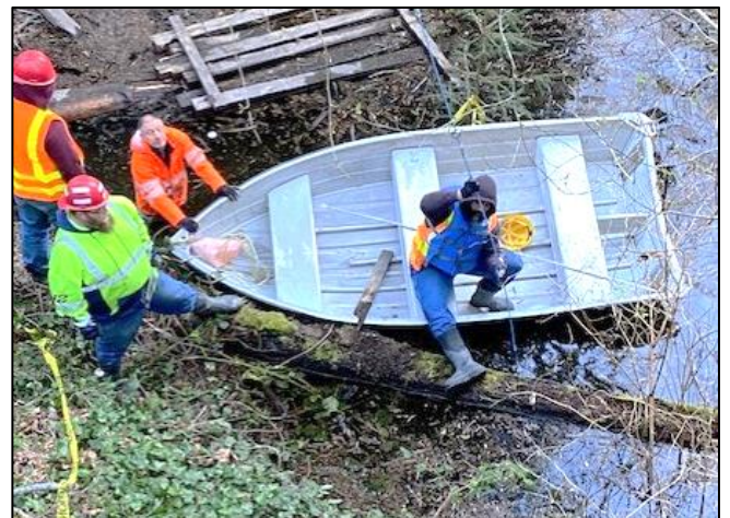
Removing the culvert blockage required the city crew to employ a boat to navigate in "Fautleroy Pond."
