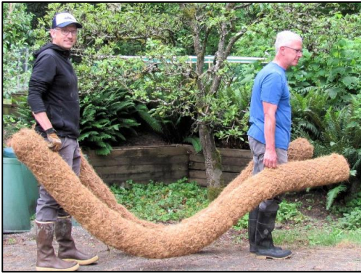
Steve Winter and Tim Wulfekuhle lugged coir logs down for Mark Sears and Pete Draughon to stake into place in the lower creek.
