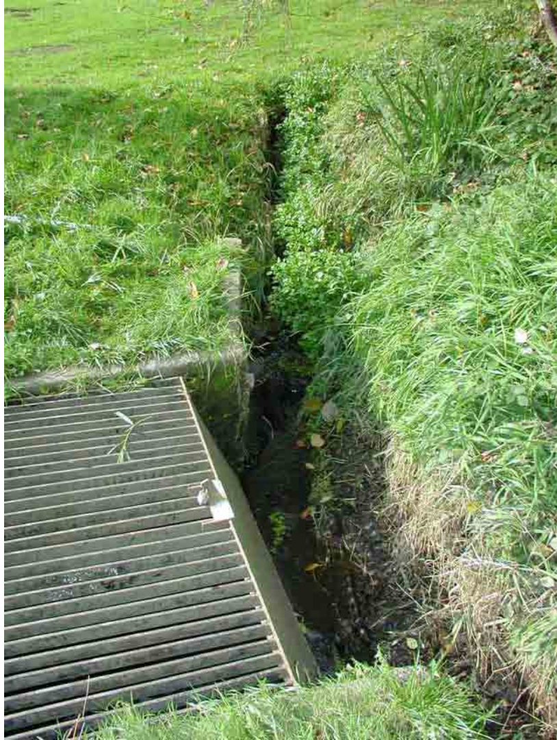
FIGURE 1.4.-- Photo taken of the culvert that Licton Springs Creek flows into at the south end of Licton Springs Park. Note there are two branches flowing into the culvert. At the time of our survey, water was only flowing in from the top branch in the photo.
