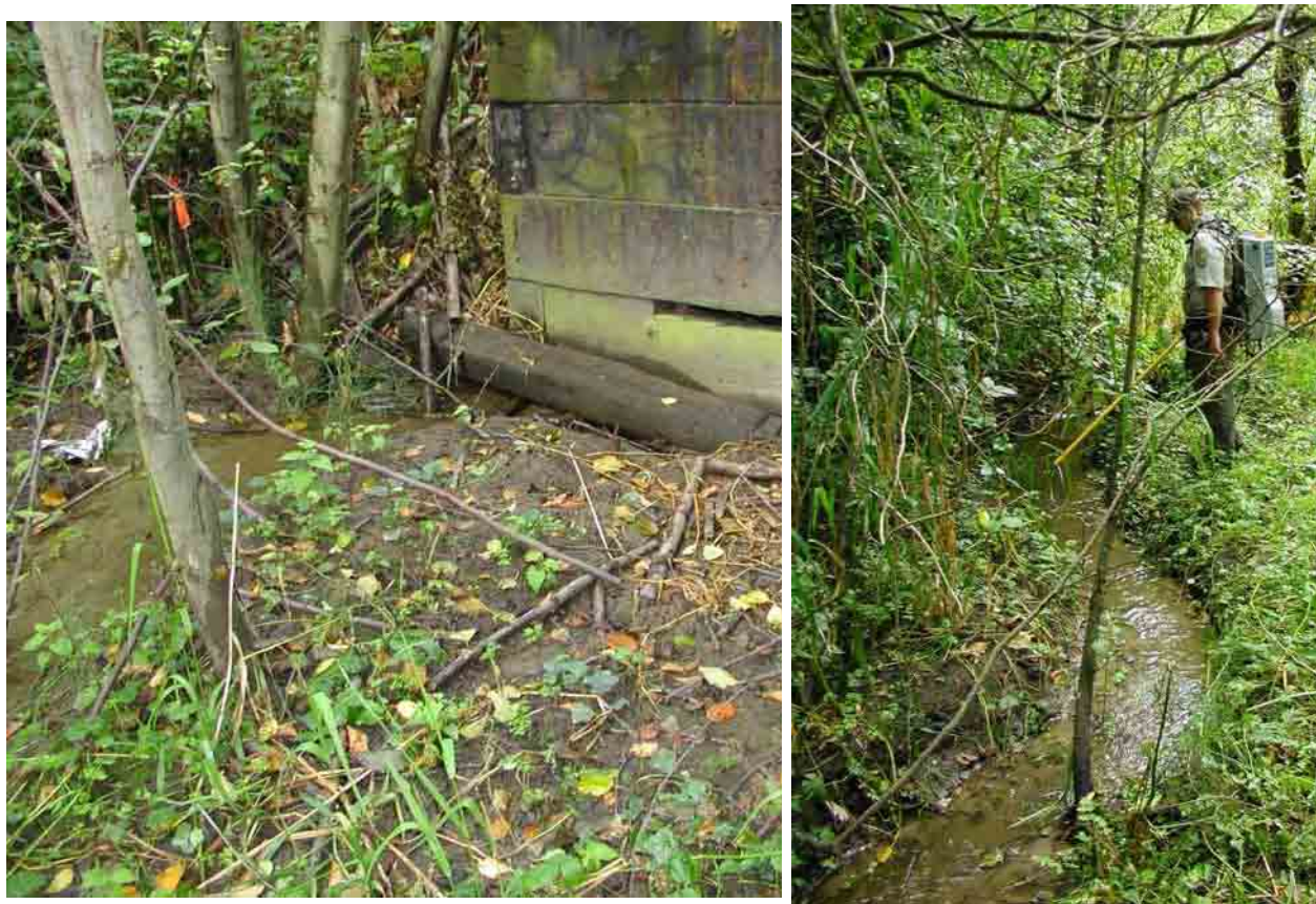
FIGURE 1.9.-- Photos of Wolfe Creek (stream system #20). The left photo was taken at the downstream end of the daylighted section where it enters into a culvert (sample location #112). The right photo shows the overall shallow depth of this stream at this site and the predominantly sand substrate.
