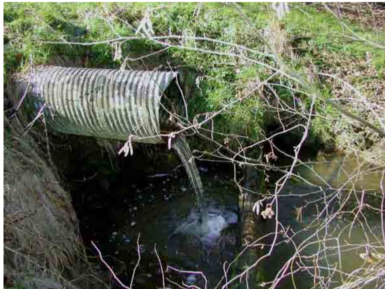
FIGURE 2.12.-- Culvert on Washington Park Creek that appears to act as a complete barrier to upstream movements of fish. Prickly sculpin and cutthroat trout were collected in the plunge pool shown but not upstream of the culvert.
