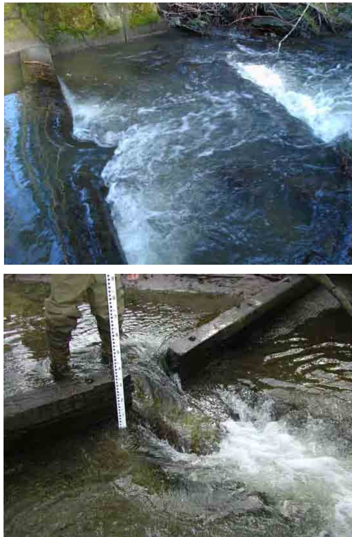
FIGURE 2.10.-- Weirs in Thornton Creek (top panel) and Piper's Creek (lower panel) that appear to act as a partial barrier to upstream movement of cottids.
