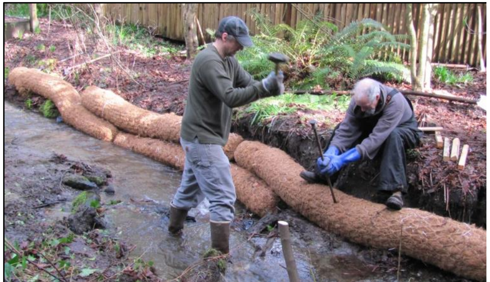
Steve Winter and Mark Harmon secure coir logs to stabilize and rebuild the bank.
